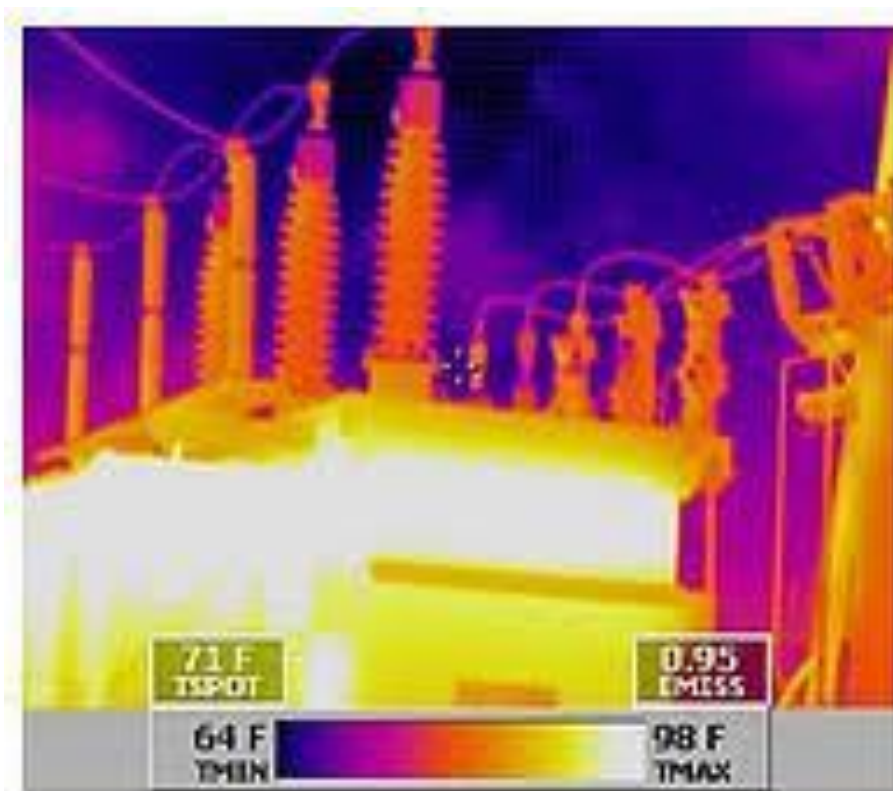
Load = Heat This Transformer Is Hot Because It Is Loaded Up
