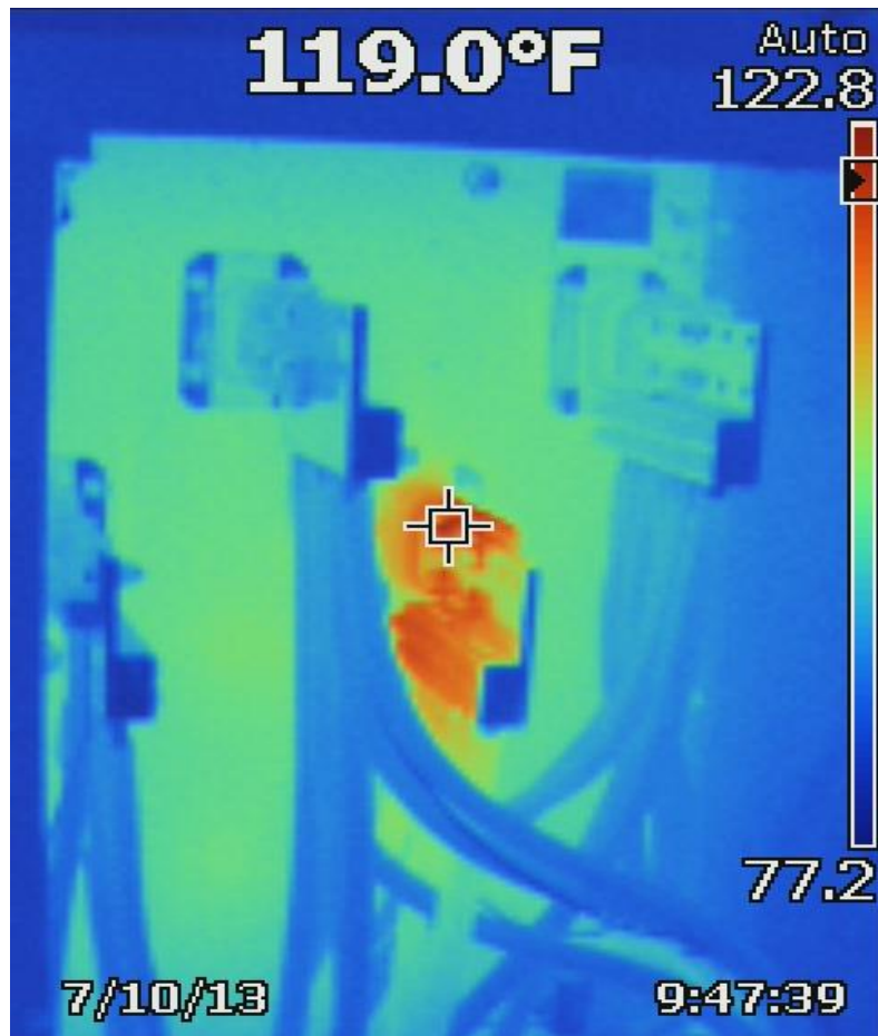
Loose Connection On 'B' Phase Spade
