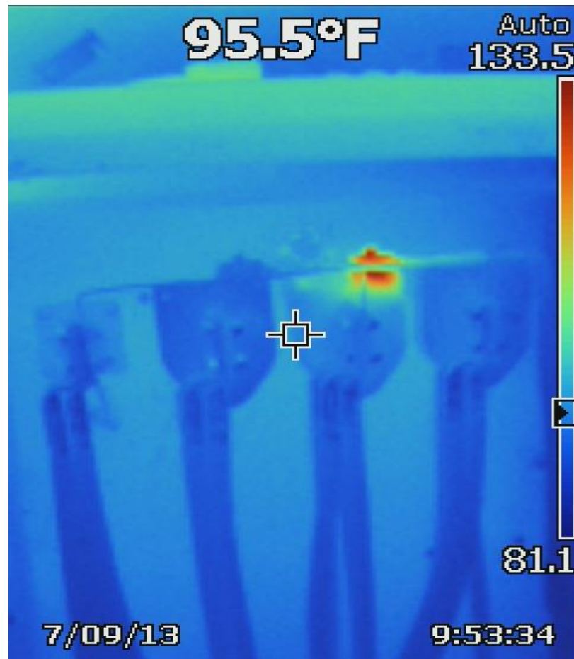
Loose Connection On 'B' Phase CT Terminals
